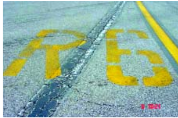
Photograph 7 Marking showing direction TWY R5.
